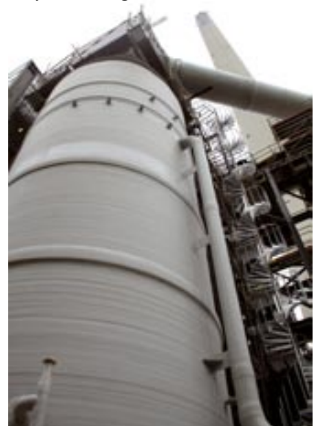
Flue gas condensation equipment at Vestforbrænding
