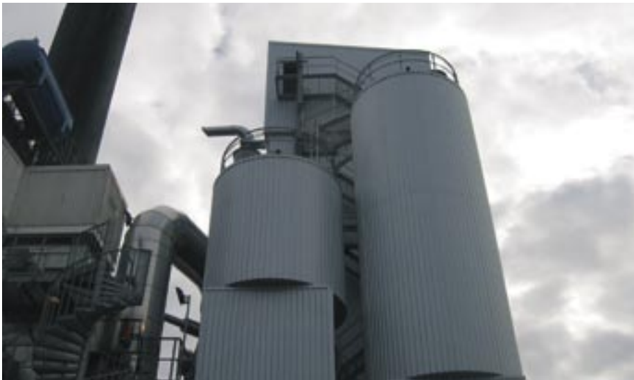
Dry flue gas treatment systems
