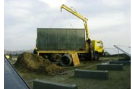
GJ Teknik assembles and installs panels for extension of the Marstal solar heating plant.
