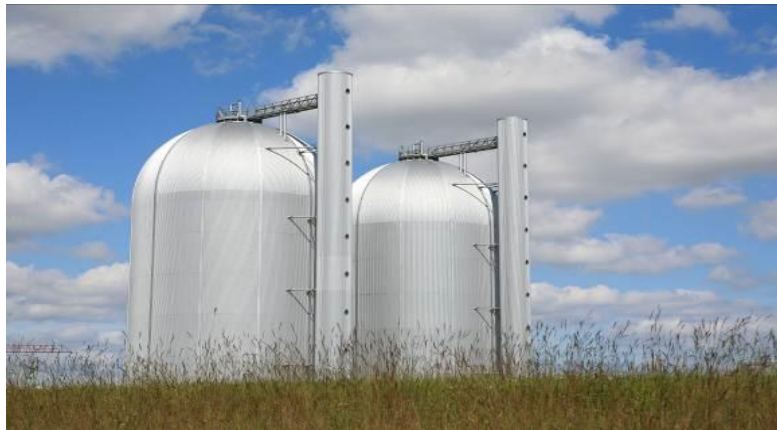
Figure 5: The two 24,000 m 3 heat accumulators of Avedøreværket.
